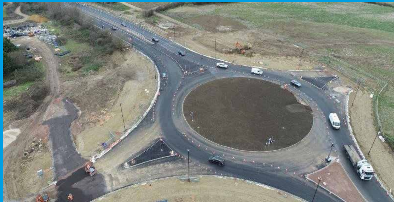
The roundabout that will join the A2300 to the Western Link Road, looking West
