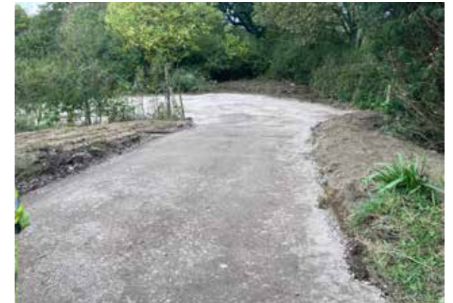
Sisk staff members volunteered for the Mid Sussex Community Garden in Cuckfield, providing their professional services to create a safe access track and space for outdoor seating.
