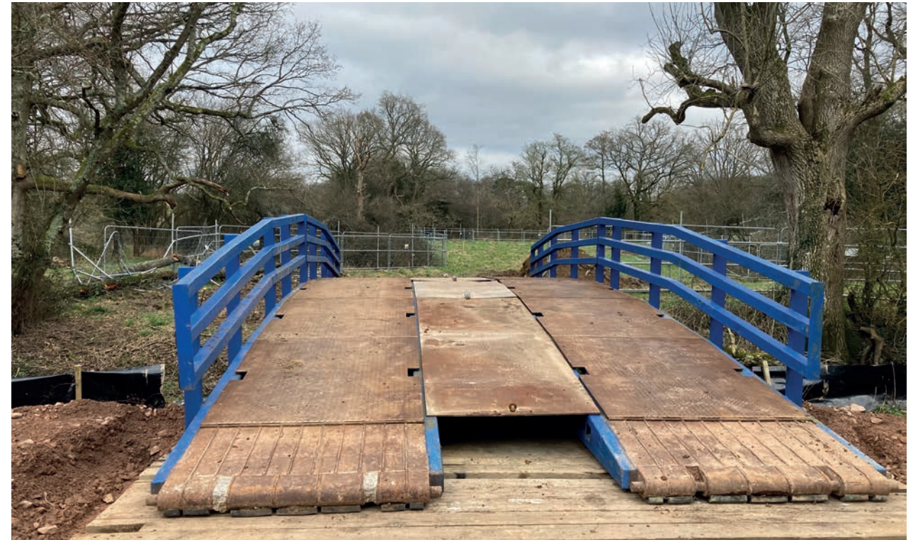
The temporary bridge provides construction traffic with access to both sides of the river to make the abutments. You can also see black reptile fencing and metal tree protection fencing which ensure the preservation of wildlife and habitat at the site.
