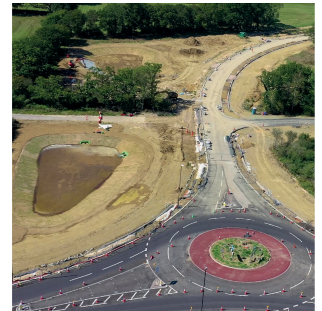
Image of the Western Link Road and south basin pond under construction
