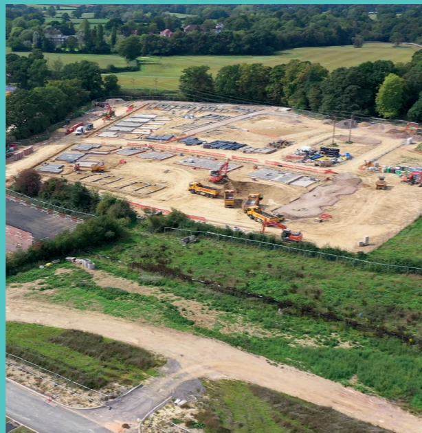
Image of the newly laid foundations at the Bellway construction site at Brookleigh
