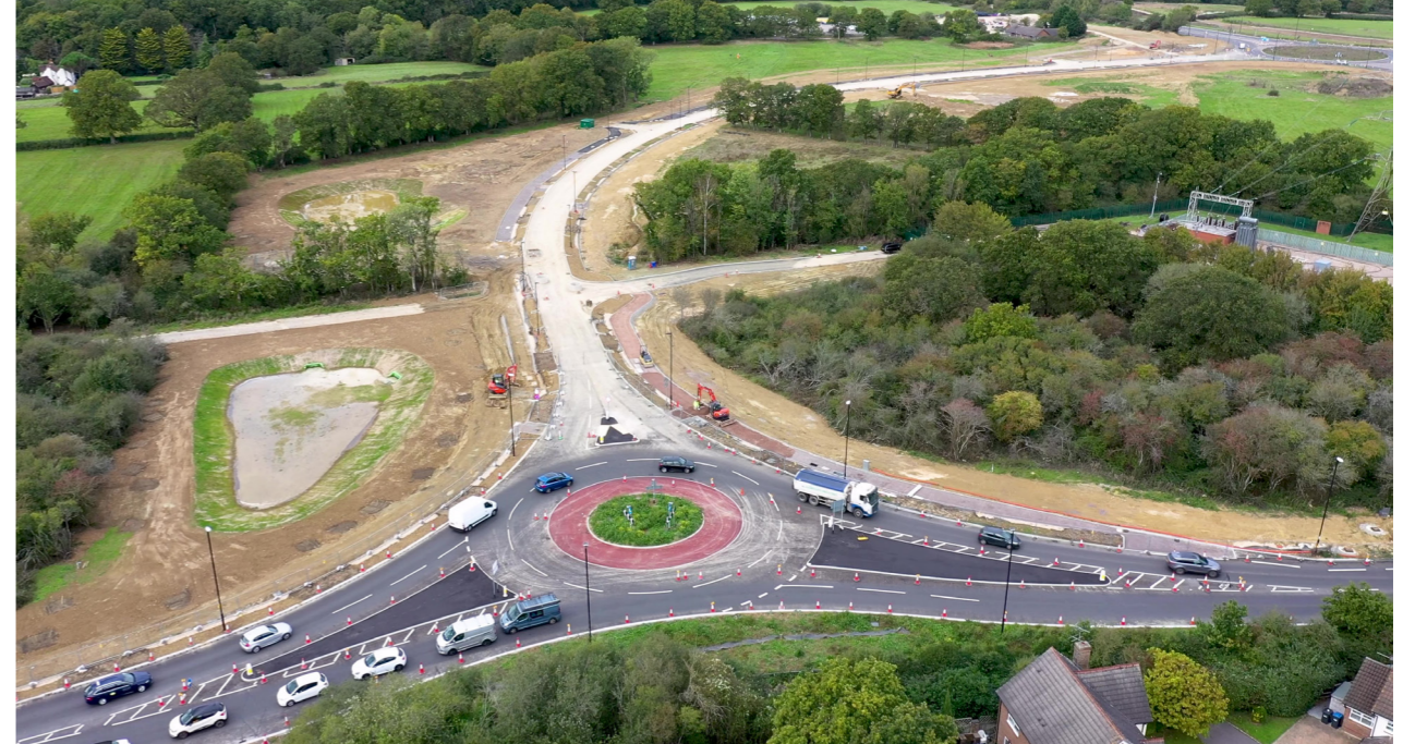
Image of the Western Link Road and new roundabout on Jane Murray Way
