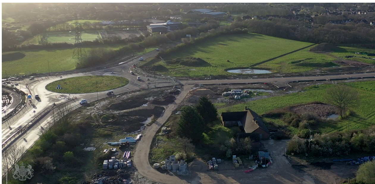
A drone image of the Western Link Road where it joins the A2300
